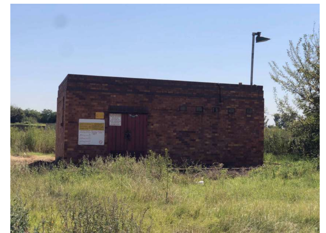
EXISTING SUBSTATION C
